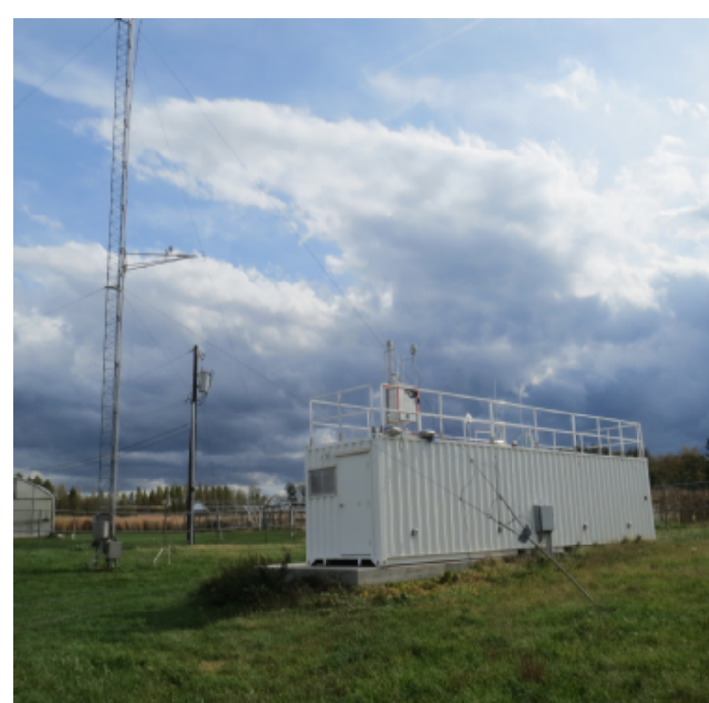
Figure 2. View of the Weather Proof Cabinet on Site
